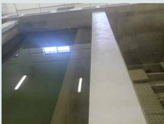
Station de pompage
